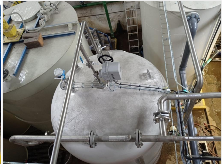
Ozone Contact Tank
